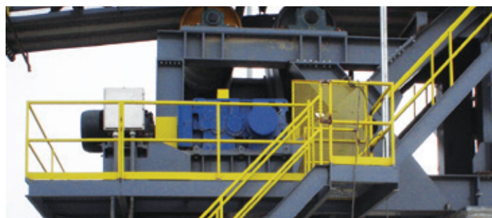
Paramax conveyor drive
