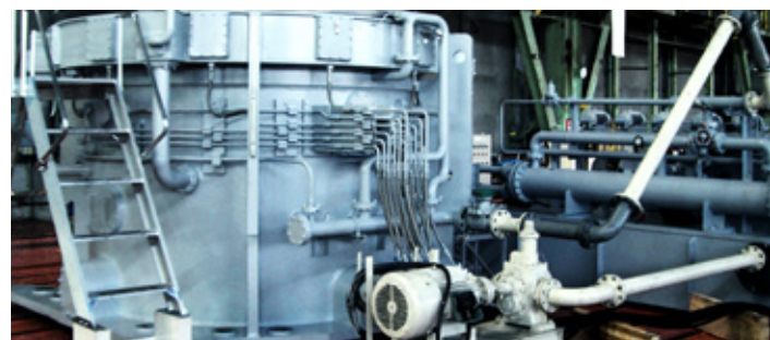
Vertical mill drive
